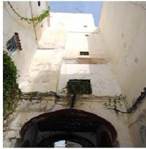
Vault ALAARS, West entry
